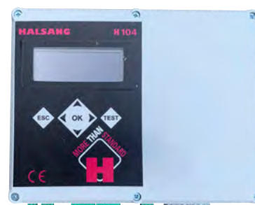
Electrical cabinet equipped with a Halsang H104 controller and frequency modulators
